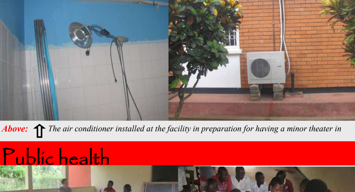
Above: ↑ The air conditioner installed at the facility in preparation for having a minor theater in
